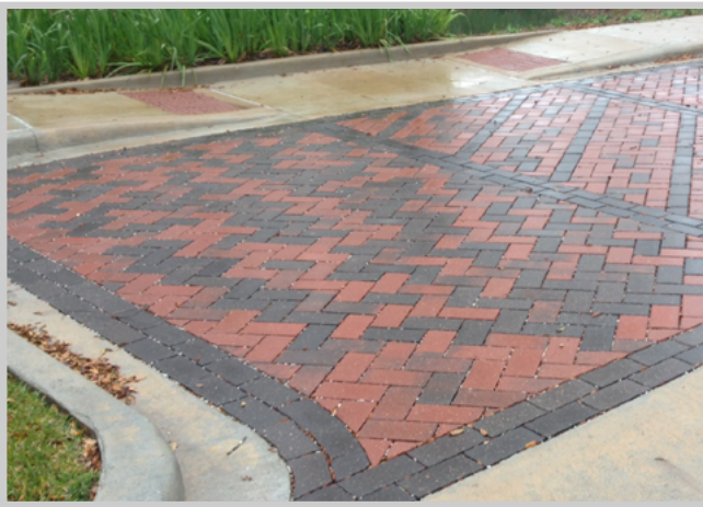
PERVIOUS PAVERS IN THE RAIN. LEAGUE CITY, TX. PHOTO COURTESY OF TCWP - TEXAS A&M AGRILIFE.
