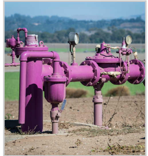
Purple pipes are used to indicate water is not potable or drinkable. (CC) FLICKR
