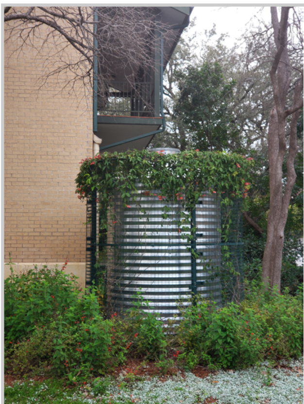
RAINWATER HARVESTING SYSTEM PHOTO COURTESY HALFF ASSOCIATES
