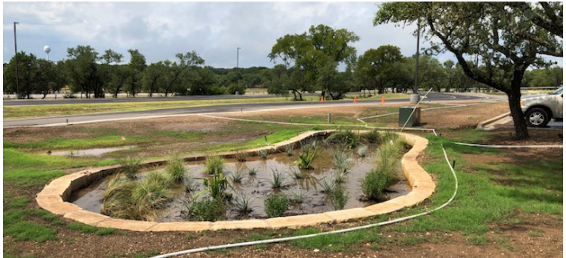
Figure 12: A rain garden after significant rainfall. Photo by Bob Farmer.
