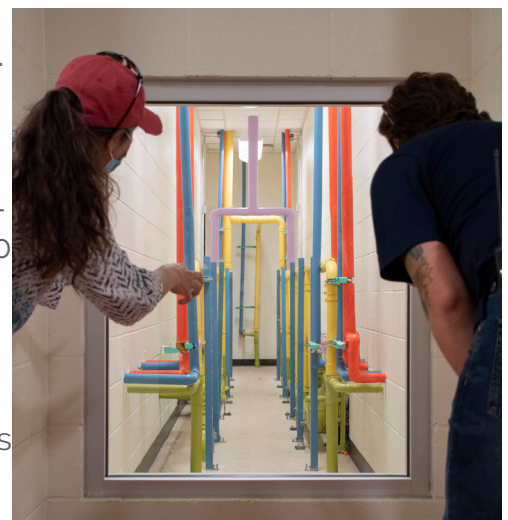
Figure 7: The plumbing window with color-coded pipes. Photo by Ray Don Tilley.
