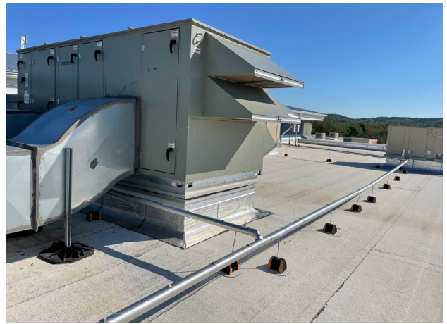
Figure 8: Condensate from 84 roof-top AC units contribute to the site harvested supply. Photo by Robin Gary.
