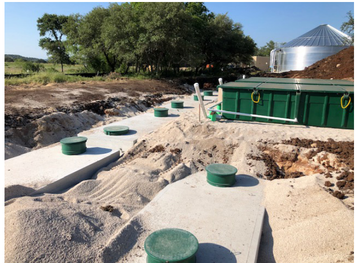
Figure 9: Components of the onsite treatment system during installation. Photo credit: Bob Farmer.
