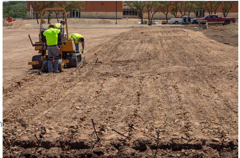
Figure 10: The subsurface, drip irrigation system being installed. Photo by Ray Don Tilley.
